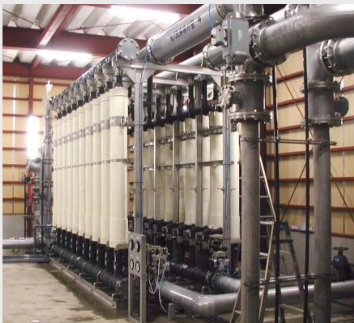
Water purification plant by membrane treatment
