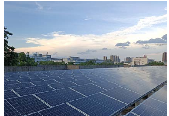
A solar power generation system of Toray Plastics Precision (Zhongshan) Ltd. (China)
