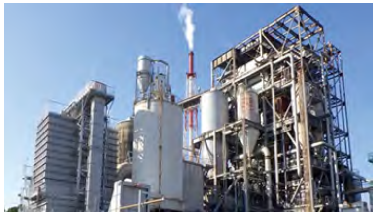
Expanded biomass fuel facilities at Toray's Tokai Plant
