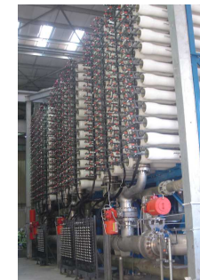
Seawater desalination plant in Algeria
