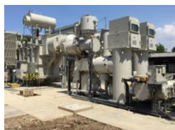
ITS power receiving and transforming equipment
