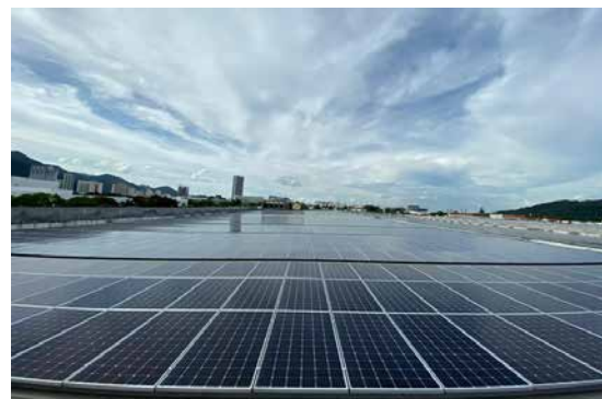
A solar power generation system of Penfabric Sdn. Berhad (Malaysia)
