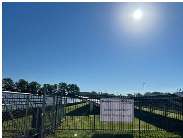
Solar panels installed on Toray Resin Co. (United States) grounds
