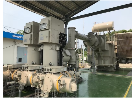
Transformer substation at P.T. Indonesia Toray Synthetics
