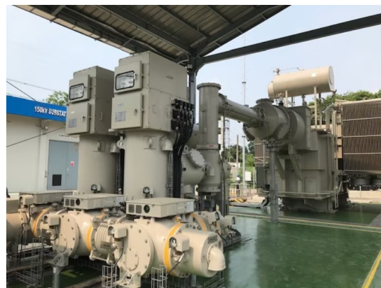
Transformer substation at P.T. Indonesia Toray Synthetics
