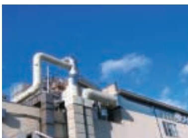
Organic exhaust gas catalytic combustion system installed at Toyo Metallizing Co., Ltd. (now Toray Advanced Film Co., Ltd.)
