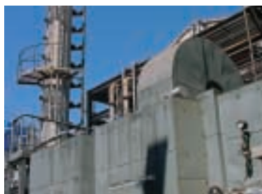
Denitrification system at the Tokai Plant
