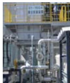
Regenerative combustion facility (2nd stage) at the Chiba Plant
