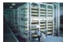
Seawater desalination plant (Okinawa)
