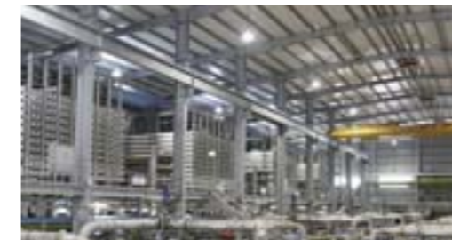
Tuas (Singapore), Reverse Osmosis Building, SingSpring Desalination Plant, Hyflux Ltd, one of the world's largest seawater reverse osmosis desalination plants Capacity: 136,000 m³/day Photograph: Hyflux Ltd (Singapore)
