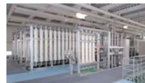
Kinuta & Kinuta-shimo Purification Plants (Tamagawa/Tokyo, Japan), one of Japan's largest filtration facilities Capacity: 88,000 m³/day Photograph: Suido Kiko Kaisha, Ltd. (Japan)
