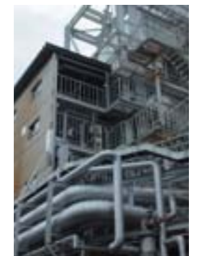
Natural gas boiler at the Mishima Plant
