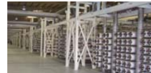
Sulaiabiya (Kuwait), the world's largest wastewater reclamation plant by membrane Capacity: 320,000 m³/day Photograph: GE-Ionics (U.S.)
