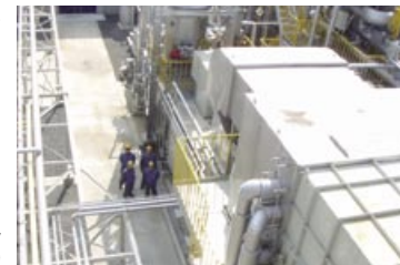
Natural gas cogeneration facility (Shiga Plant)
