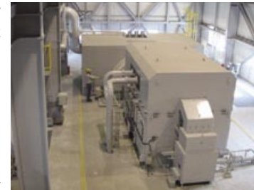
Steam turbine generator
