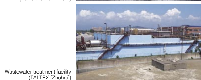
Wastewater treatment facility (Penfabric No. 4 Plant)
