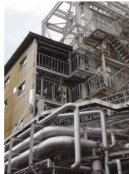
Natural gas boiler at Mishima Plant
