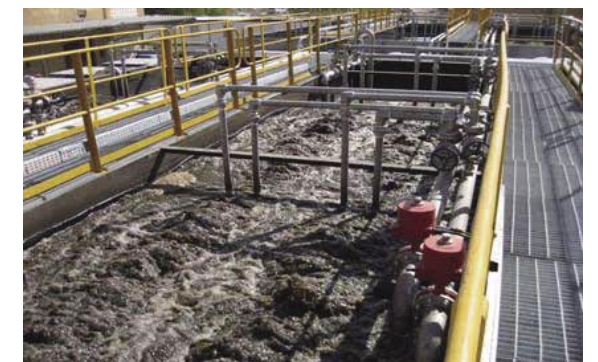
The AI Ain Sewage Reclamation Plant in UAE using Toray's submerged membrane modules for membrane bioreactors
