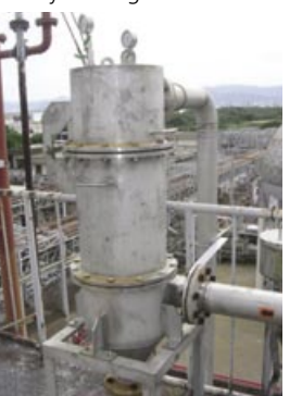
Organic exhaust gas recovery facility installed at Toray Plastics (Malaysia) Sdn. Berhad
