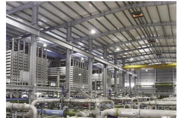
The largest desalination plant in the Pacific Rim—the SingSpring Desalination Plant, Tuas, Singapore Photo courtesy of Hyflux Ltd.
