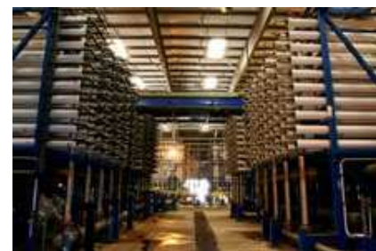
Seawater desalination plant in Trinidad and Tobago
