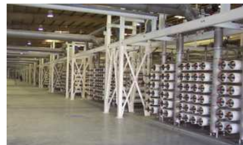
Wastewater reuse plant in Kuwait that uses Toray's low fouling RO membrane
