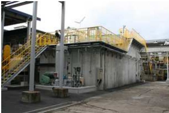
New MBR wastewater treatment facility at the Shiga Plant
