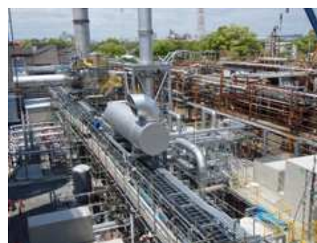
Cogeneration facility at the Nagoya Plant
