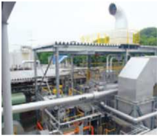
Gas boiler at Toray's Gifu Plant
