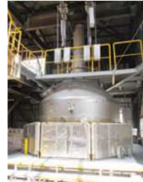
N 2 O catalytic cracking facility at Toray's Tokai Plant
