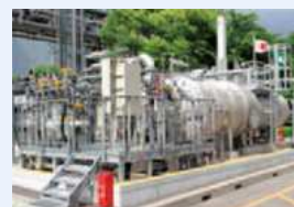
Boiler that uses byproduct oil as fuel
