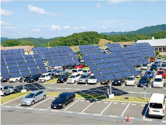
Tracking photovoltaic system developed by Fujipream Corporation. The elevated system enables the space underneath the panels to be used for other purposes. Solar panels automatically track the sun by calculating its position, generating power more efficiently than a fixed panel system.
