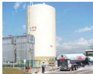
Cogeneration facilities at Toray Battery Separator Film Co., Ltd.
