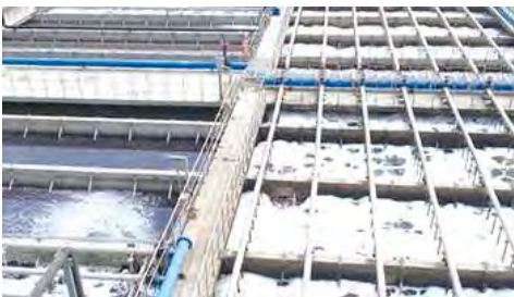
Wastewater facility at Toray Sakai Weaving & Dyeing (Nantong) Co., Ltd.
