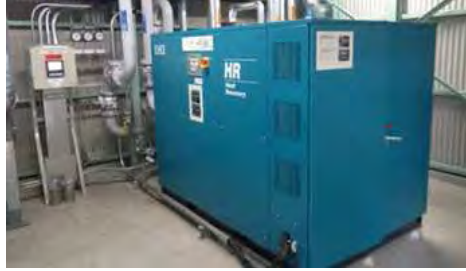
Small-scale binary power generation system installed at Toray's Tokai Plant
