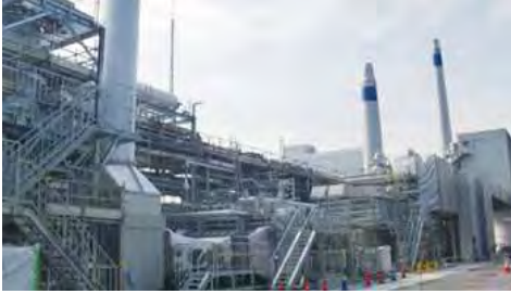
Cogeneration facilities at Toray's Mishima Plant
