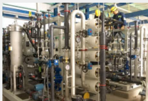
Water treatment facilities at a group company in Mexico
