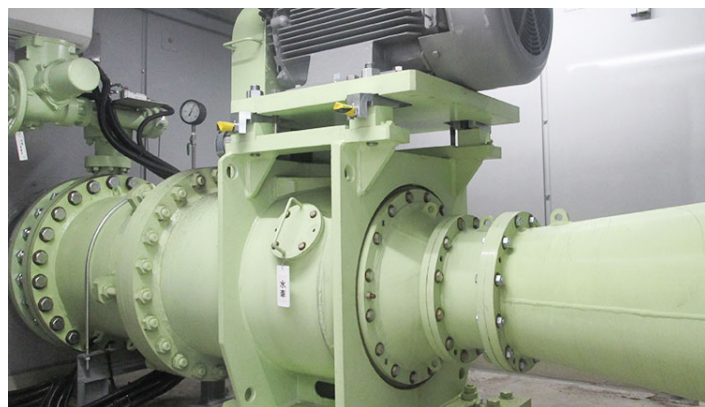
Small hydroelectric power generator at Toray's Nagoya Plant
