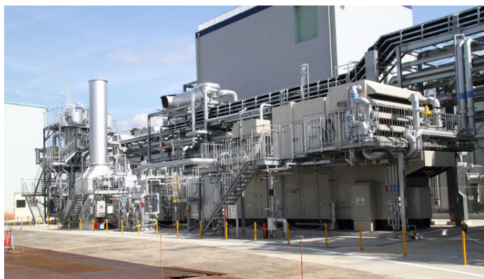
Gas cogeneration system at Toray's Mishima Plant
