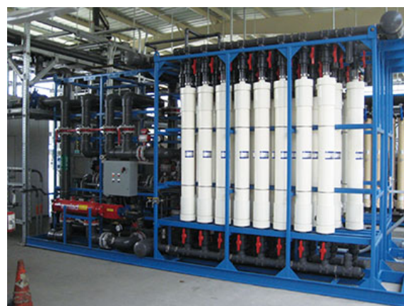
Pilot of Toray's UF membrane
