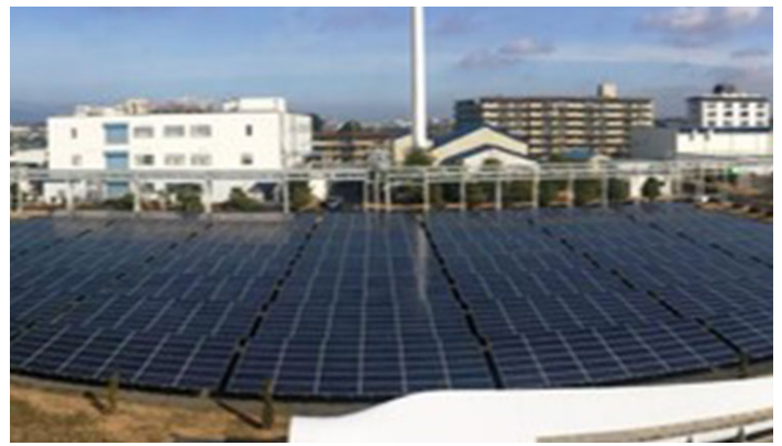
Solar power generation system at Toray's Seta Plant
