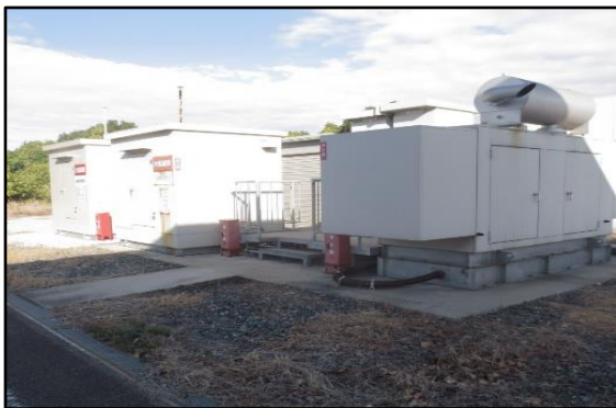
Elevated installation of an emergency generator
