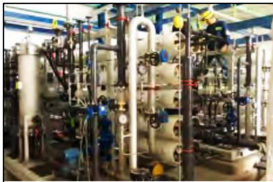
Reuse of plant wastewater using water treatment membranes
