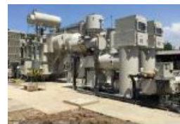
ITS power receiving and transforming facility
