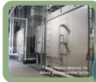
Toray Plastics (America), Inc. Operation of natural gas cogeneration facility started
