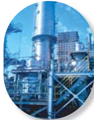
Toray Tokai Plant N 2 O thermal decomposition facility
