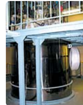
Organic exhaust gas distillation recovery system installed at Toray Ehime Plant.
