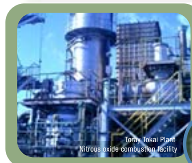
Toray Tokai Plant Operation of N 2 O thermal decomposition facility started
