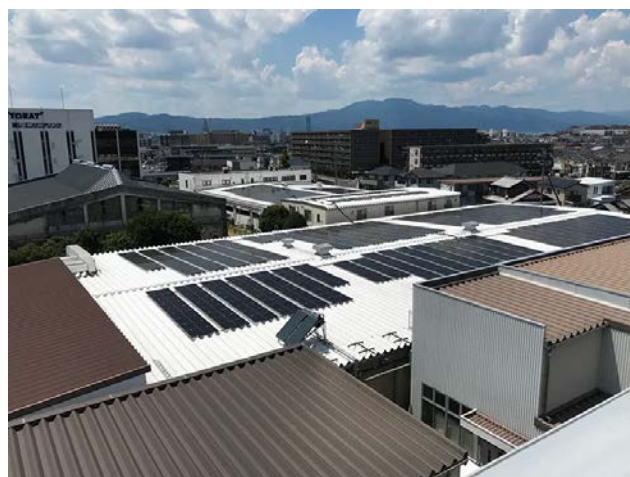
Solar power equipment at Toray Precision Co., Ltd.
