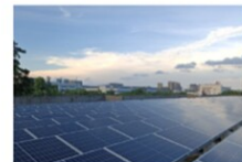
TPPZ installed with solar power generation facilities in FY 2020
