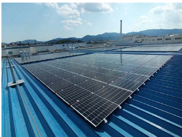
Solar power equipment at Toray Industries Seta Plant No. 3
