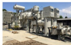
Power receiving and transforming equipment at ITS
